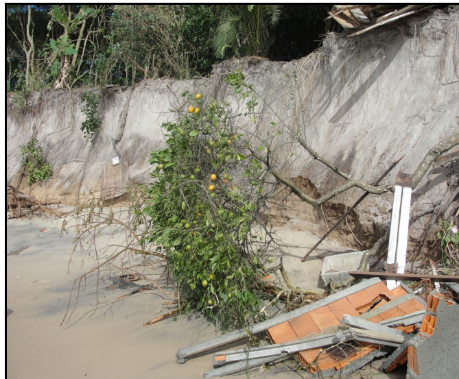
Photo 2. Coastal erosion on the beach of Armação in the Southeast coast of the island of Santa Catarina .
